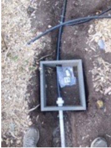
1" HDPE main originates in box
